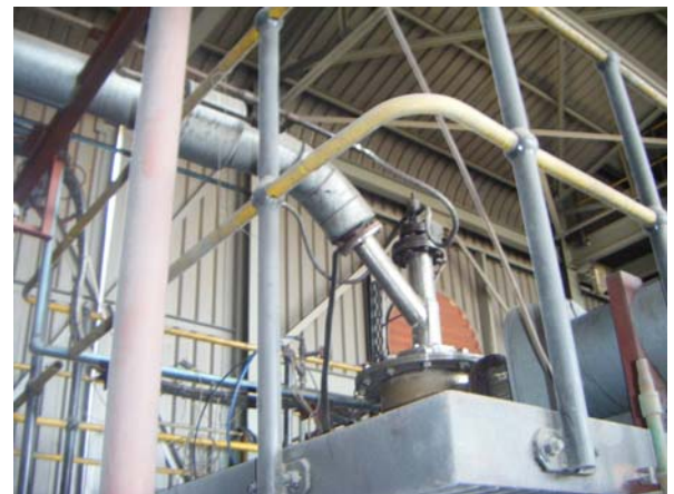
Figure 3d: Top floor shows the coal pipe to the burner
