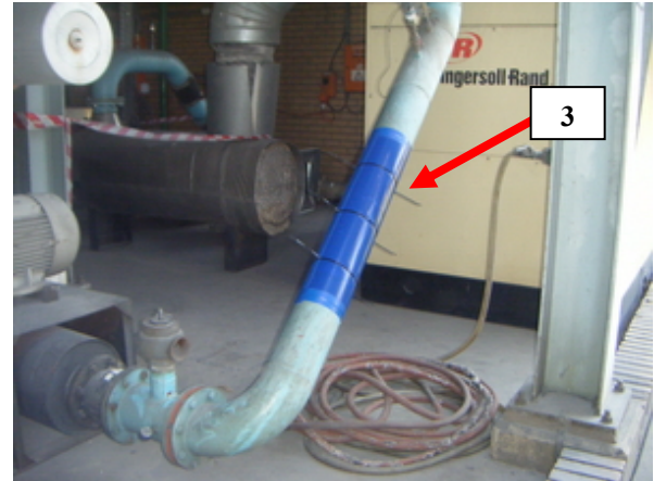
Figure 3h: XPlate™ installation site at the secondary air pipe after the blower
