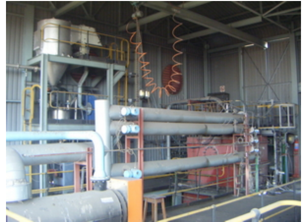
Figure 3c: Top floor shows the secondary air pipe and the combustion reactor
