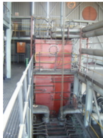
Figure 3e: Combustion chamber
